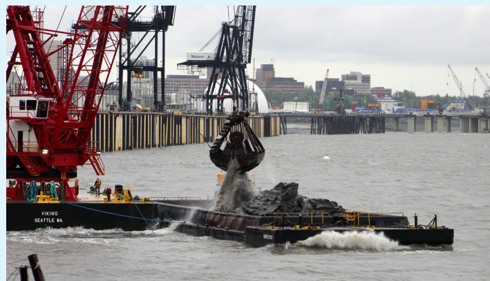
NES1 marine-based dredging widens the shipping canal making it safer for vessels to dock at the Cargo Terminals.
